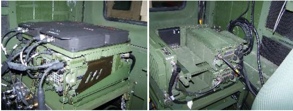
Figure 12. Examples of hardware installations that would be SAVE compliant
